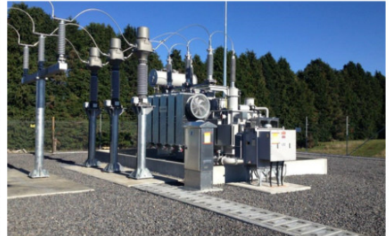
OKN Substation 110/33kV Transformer T2
