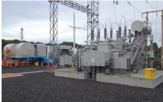
NPK 110/33kV Transformer T1
